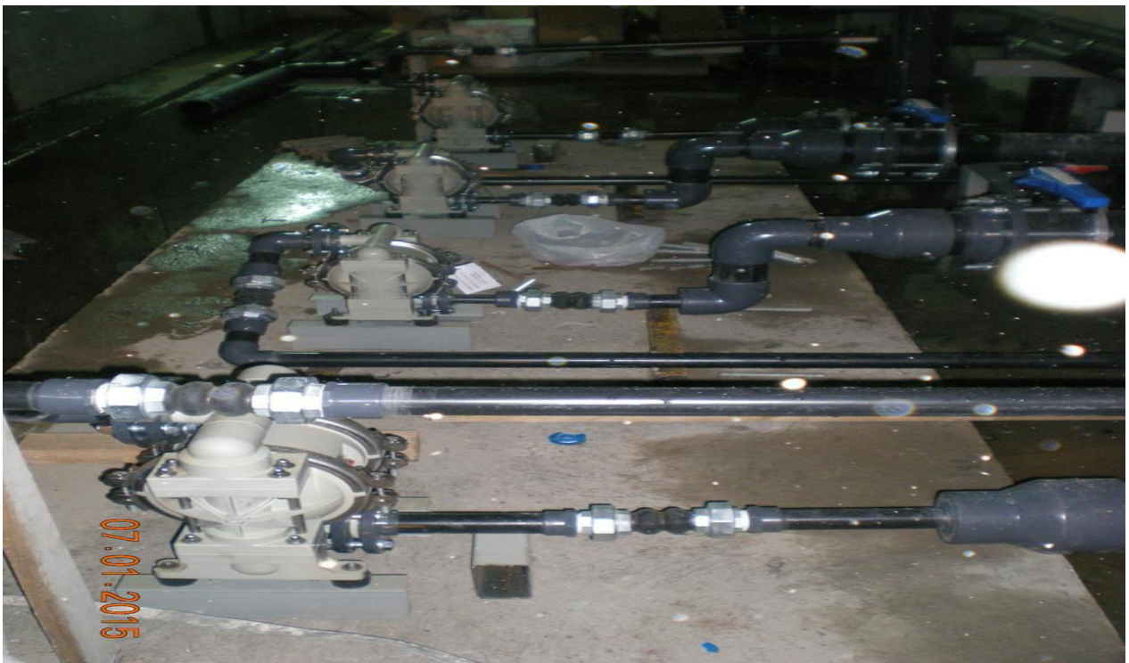
Acid and Alkaline Basin Transfer Pumps
