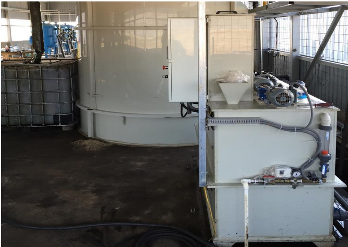
Polyelectrolyte Dosing Units
