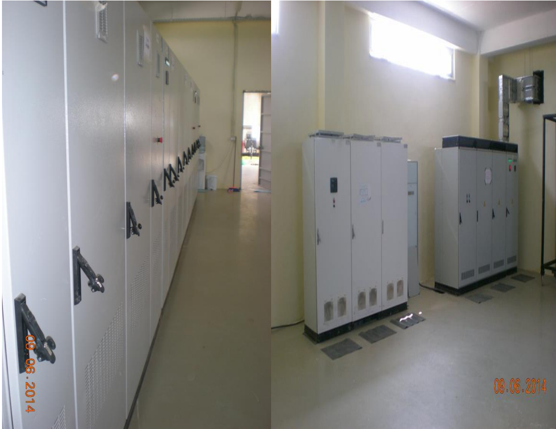
MCC Panel to Electric Cabinet
