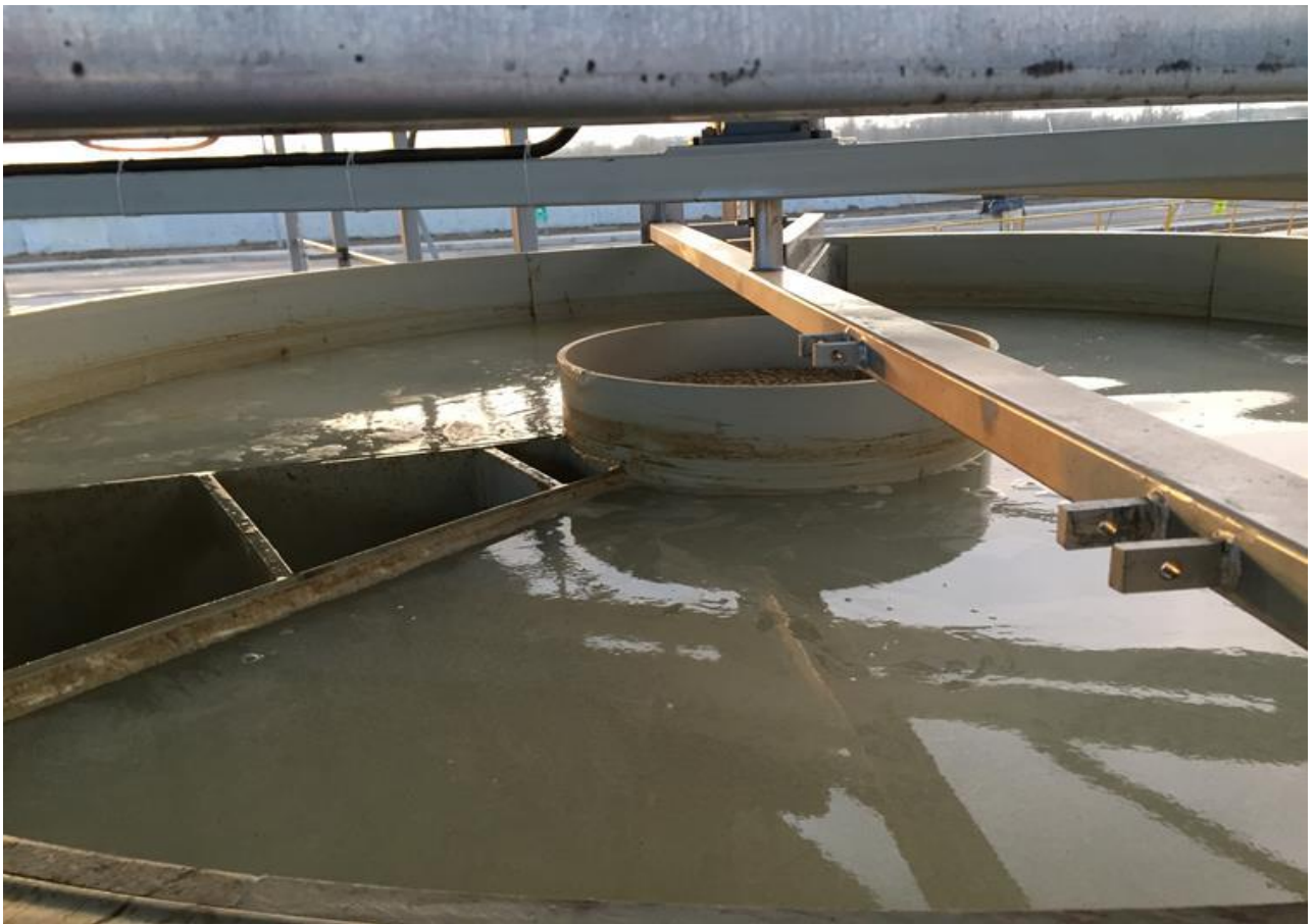
DAF (Dissolved Air Flotation ) System For Removed to Rolling Mill Oil by Water
