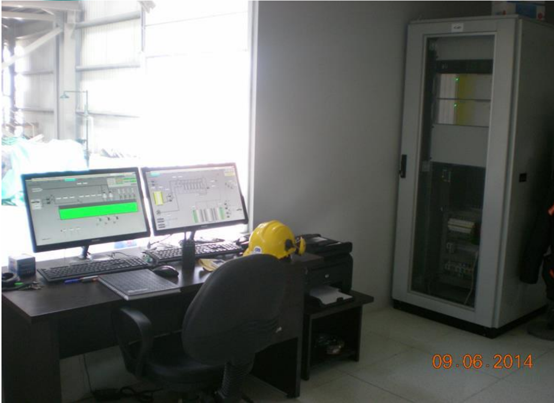
PLC Panel and Operation Pull Pit
