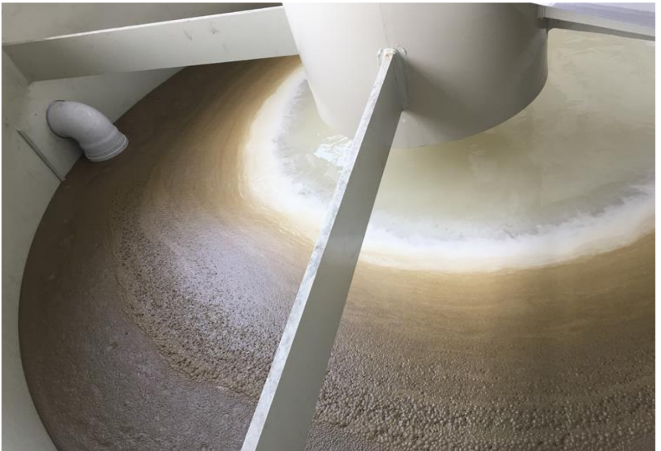
DAF (Dissolved Air Flotation ) System For Removed to Rolling Mill Oil by Water
