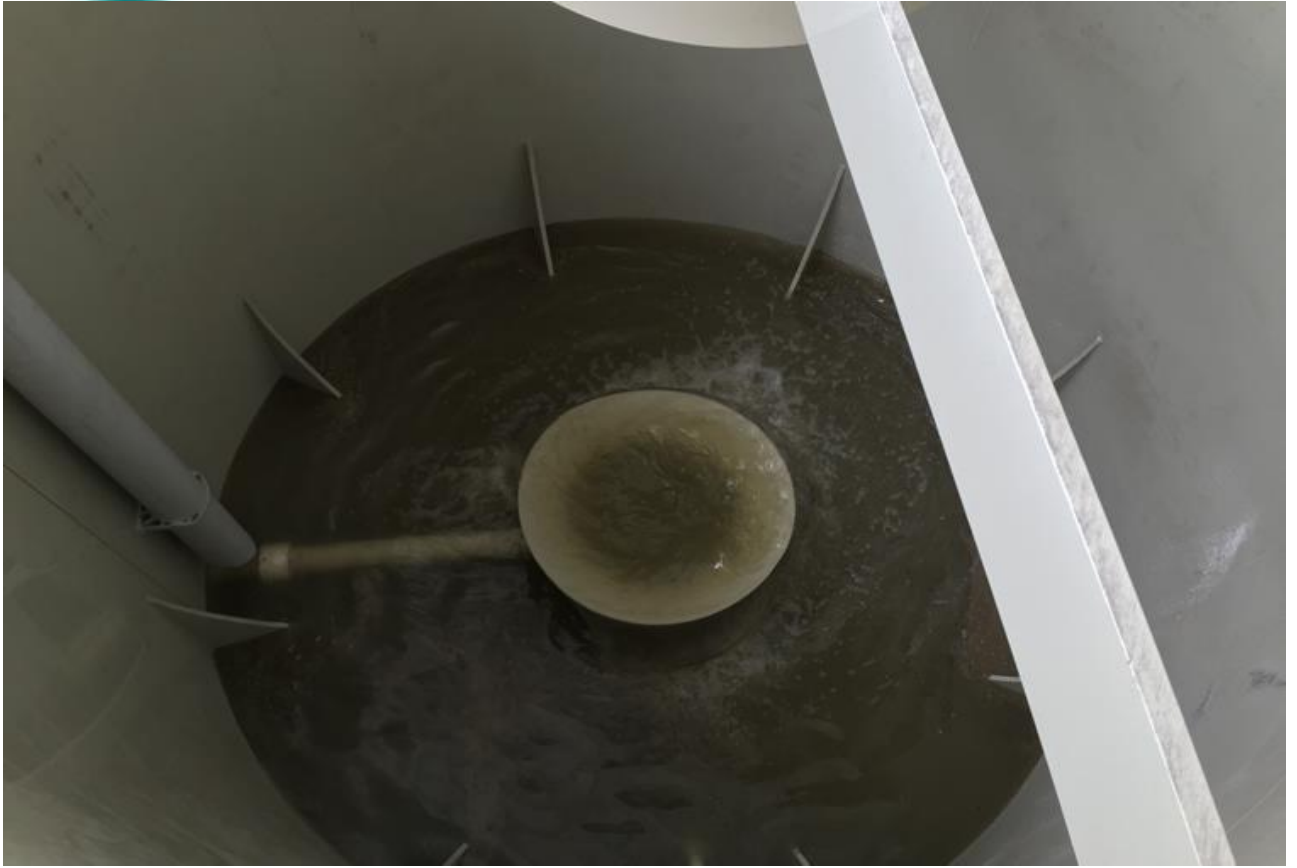
DAF (Dissolved Air Flotation ) System For Removed to Rolling Mill Oil by Water
