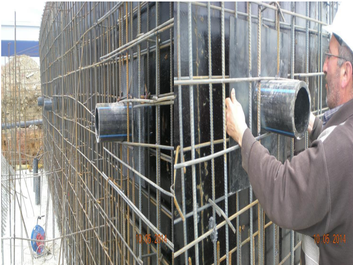
Pump Section Embedded Plate
