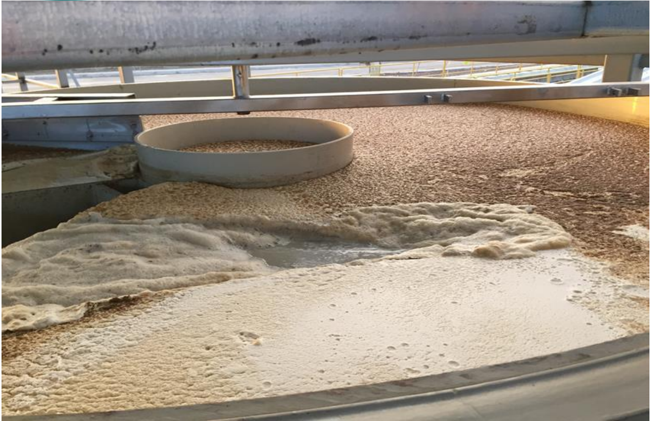
DAF (Dissolved Air Flotation ) System For Removed to Rolling Mill Oil by Water
