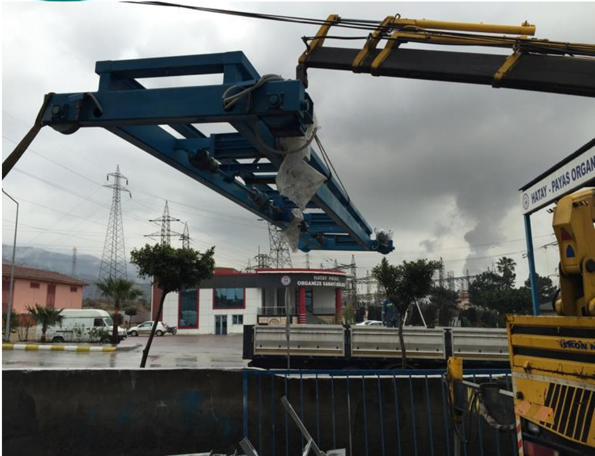
Settling Basin Scrapper Bridges
