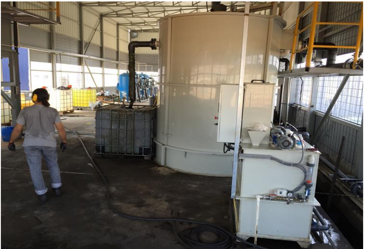
DAF (Dissolved Air Flotation) and Polyelectrolyte Dosage Systems
