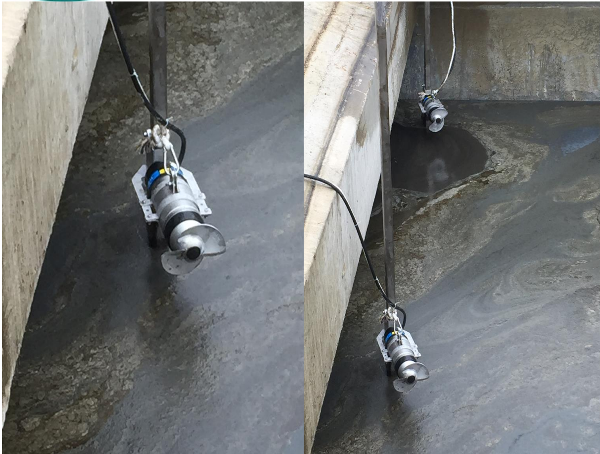
Settling Basin Rapid Mixers
