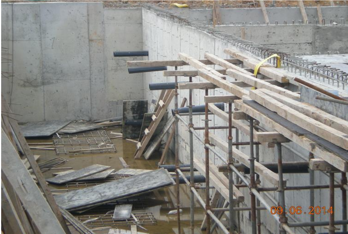
Water Basin Pump Section Pipes
