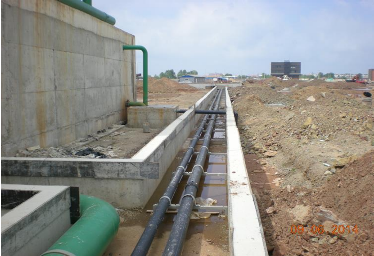
Chemical Treatment Plant Inlet Pipeline
