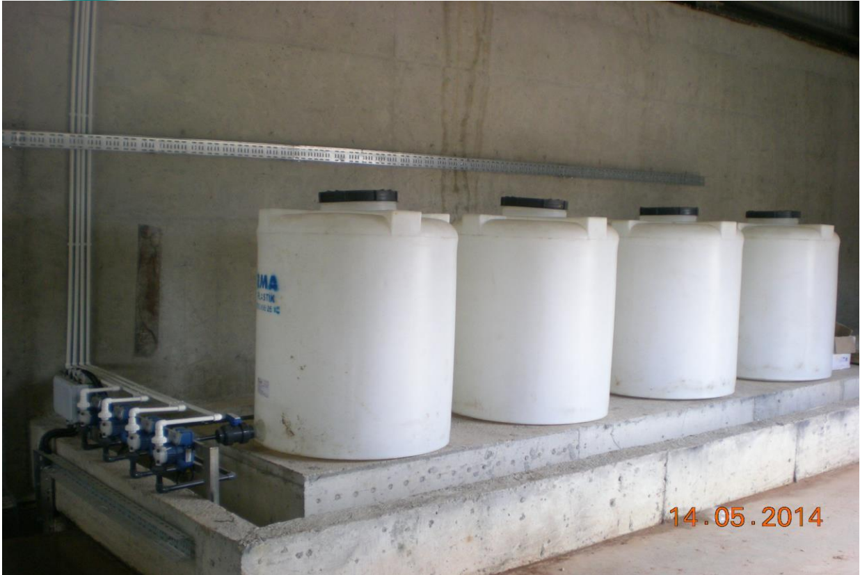
Chemical Dosing Units
