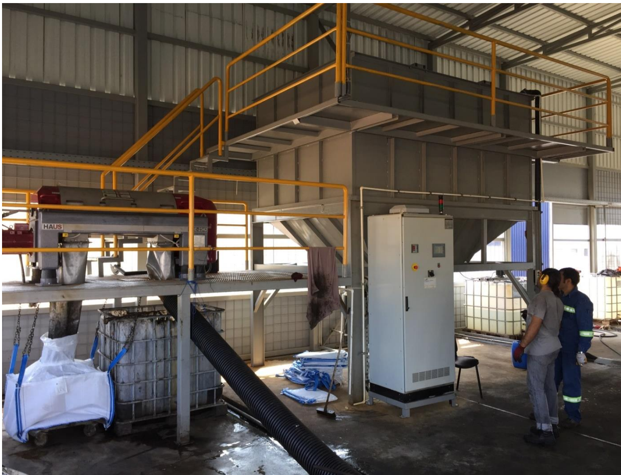
Sludge Thickener Decanter and Tank
