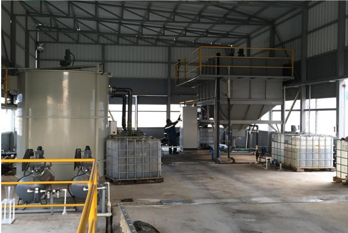
Chemical Treatment Plant Inside Hall
