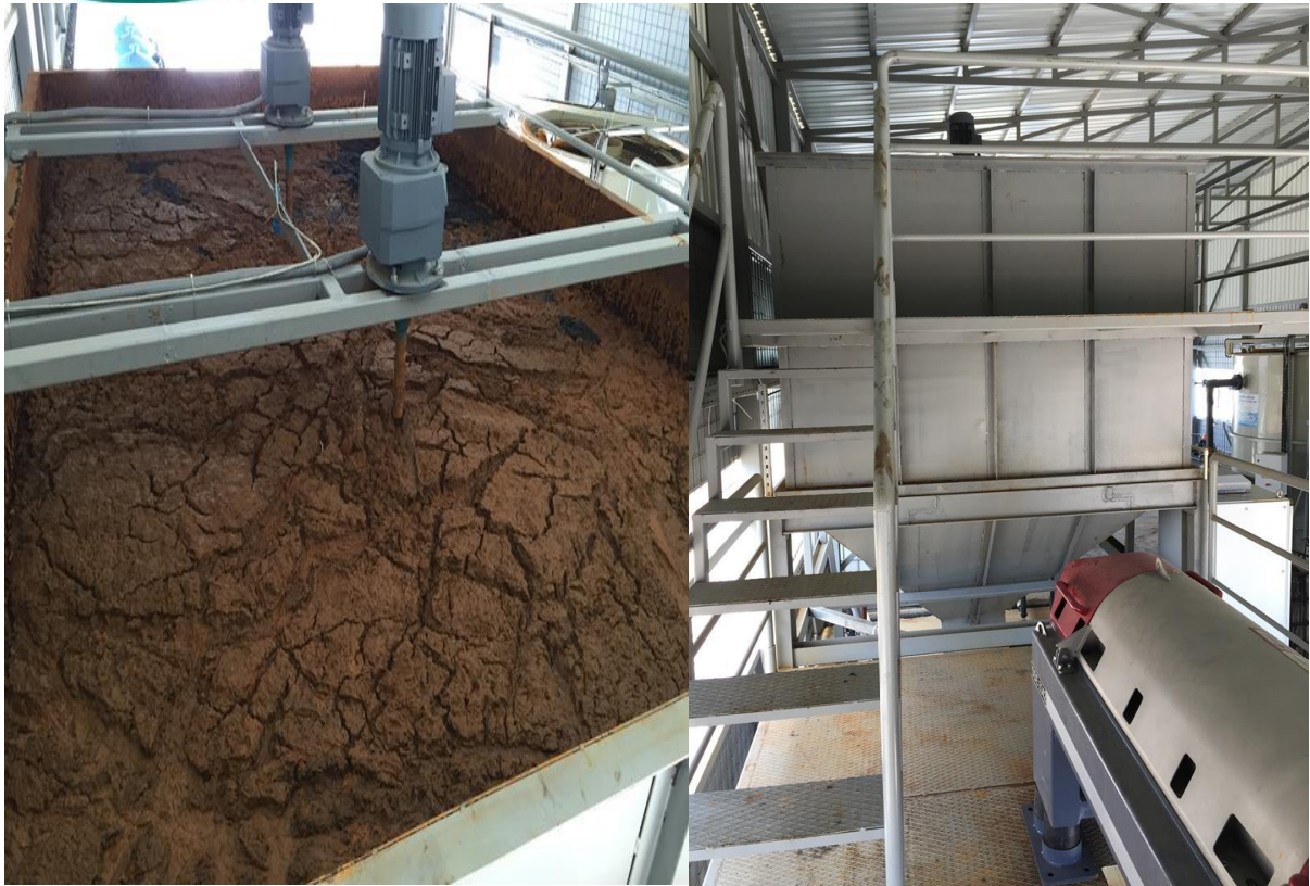
Sludge Thickener Mixers and Tank
