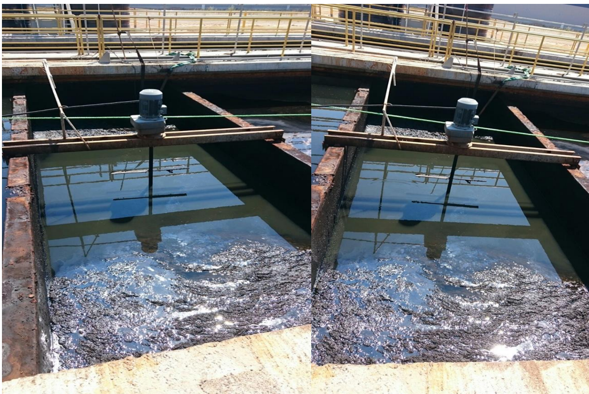
Settling Basin Slow Mixers
