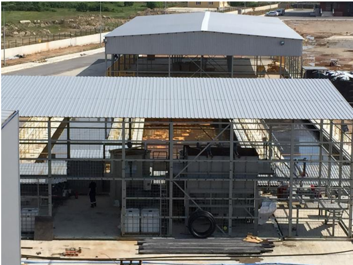
Chemical Treatment Plant General Appearance
